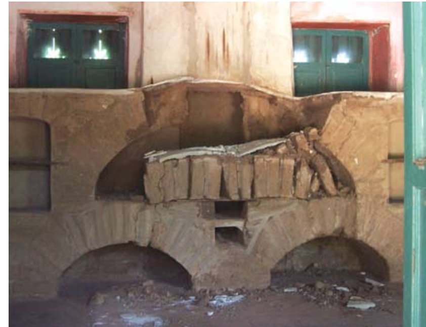
The Casa de Adobe's kitchen stove, built entirely of adobe bricks, collapsed due to water leaks in February 2005.
