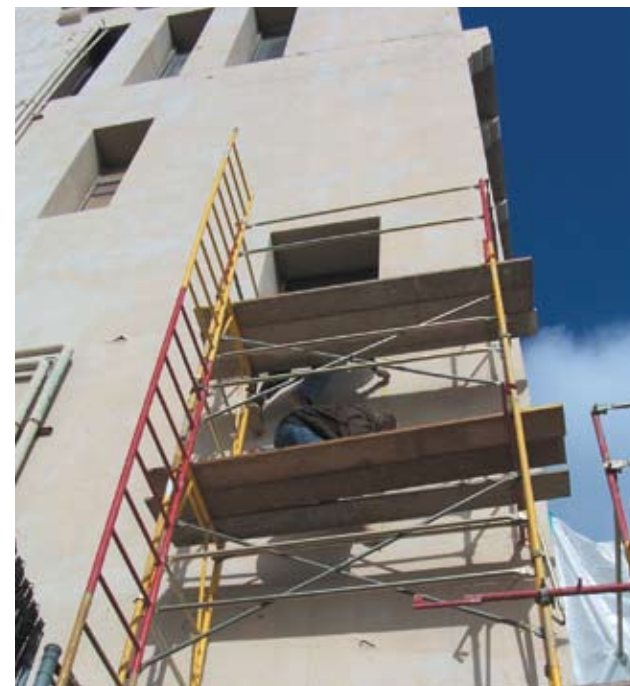
Tests were conducted in spring 2007 to determine the best method for removing and replacing plaster, in advance of repairing structural cracks in the Caracol Tower.
