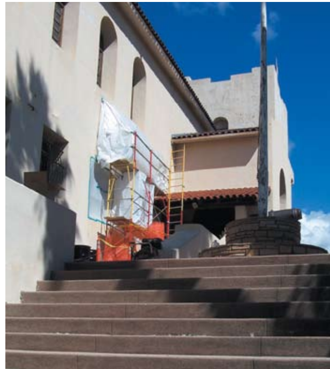
The building's exterior is in poor condition. Plaster in many locations is deteriorating due to cracking and water intrusion.
